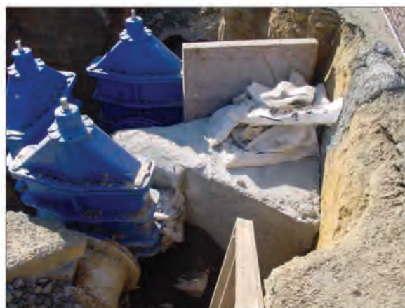
Figure 6.2 - Concrete thrust block, correctly oriented to transfer the hydraulic thrust to the specially trimmed undisturbed soil of the vertical trench walls perpendicular to the load.
