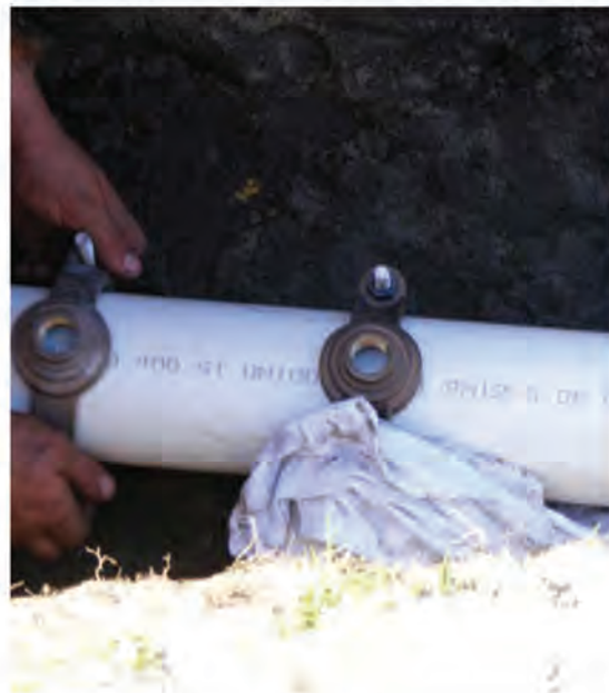
Figure 7.7 – Series 1 PVC-U pressure pipe with twin tapping saddles. Note minimum spacing between tapping saddles.
