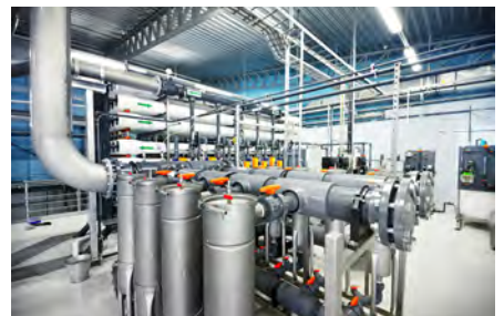
Water Pump Station
